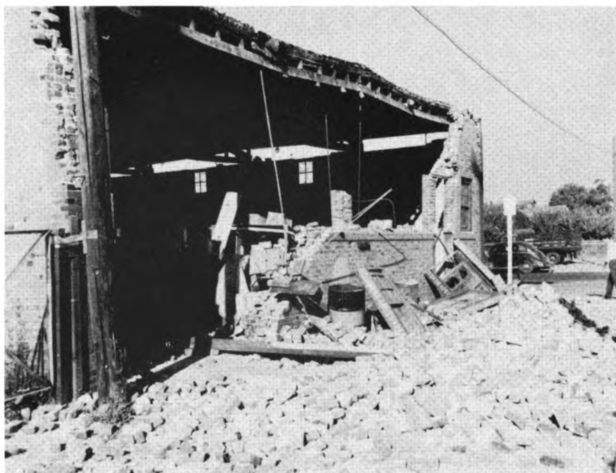
Photo No. 35—Salvation Army storeroom in Bakersfield on Sumner and Kings Streets. Brick construction; windows and doorways add to instability of a nonreinforced wall. Photo by The Bakersfield Californian.
