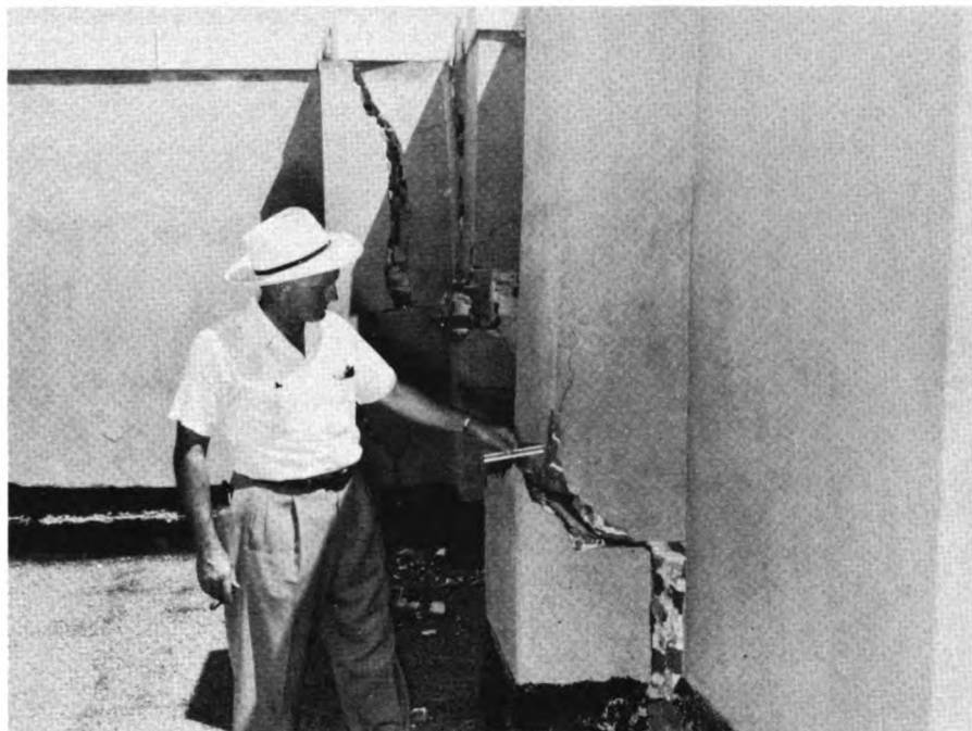
Photo No. 33—Kern County Courthouse roof showing failure of northeast corner of nonreinforced parapet. Brick construction with plaster coat. Steel column extends only to the roof. Photo by The Bakersfield Californian .
