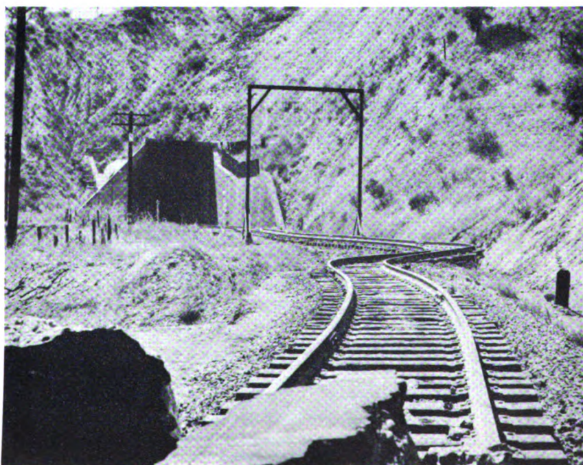
Photo No. 18—Rails twisted by compression between Southern Pacific Tunnels 3 and 4 about one mile south of Caliente. Photo by Southern Pacific Company.
