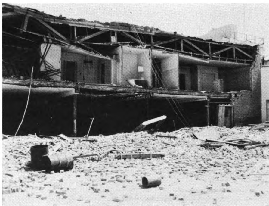
Photo No. 34—Eye Street apartment in Bakersfield. Complete collapse of brick rear wall. Photo by The Bakersfield Californian .
