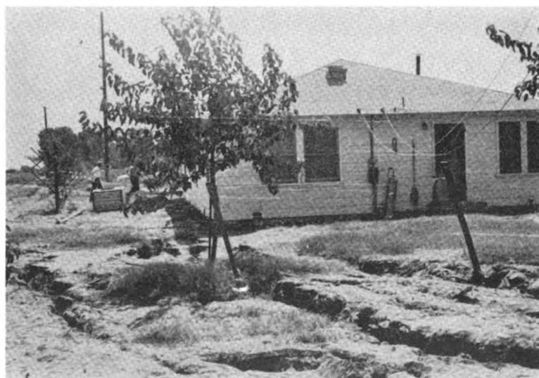
Photo No. 8—Cracking of ground about three miles southwest of Arvin. Cracks turn and go under house, and though chimney fell and house was slightly damaged it still stands. Photo by Division of Architecture.
