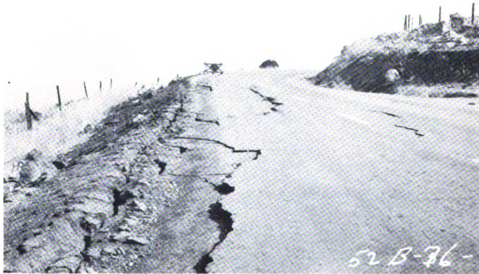
Photo No. 14—Road cracking and slumping on the Arvin-Tehachapi road. Photo by Division of Highways.
