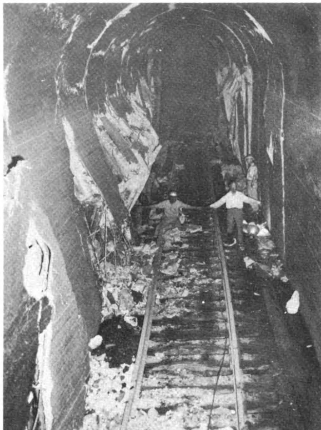
Photo No. 23—Facing south in Southern Pacific Tunnel 5. Compression of east wall toward west. Photo by Southern Pacific Company.
