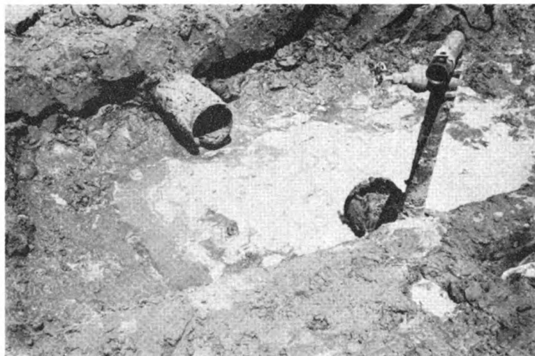
Photo No. 7—Facing north, steel water line pipe separated about 17 miles south of Bakersfield, and one-half mile east of U. S. Highway 99.
