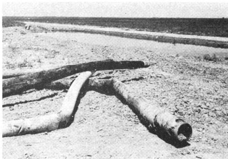
Photo No. 3—Replaced oil line pipes about 15 miles south of Bakersfield which have been bent, twisted, telescoped up to 36 inches and separated up to 55 inches. Pipes are constructed of five-sixteenth inch steel and range from six to 12 inches in diameter. Lines are generally placed from two to three feet below the ground surface.
