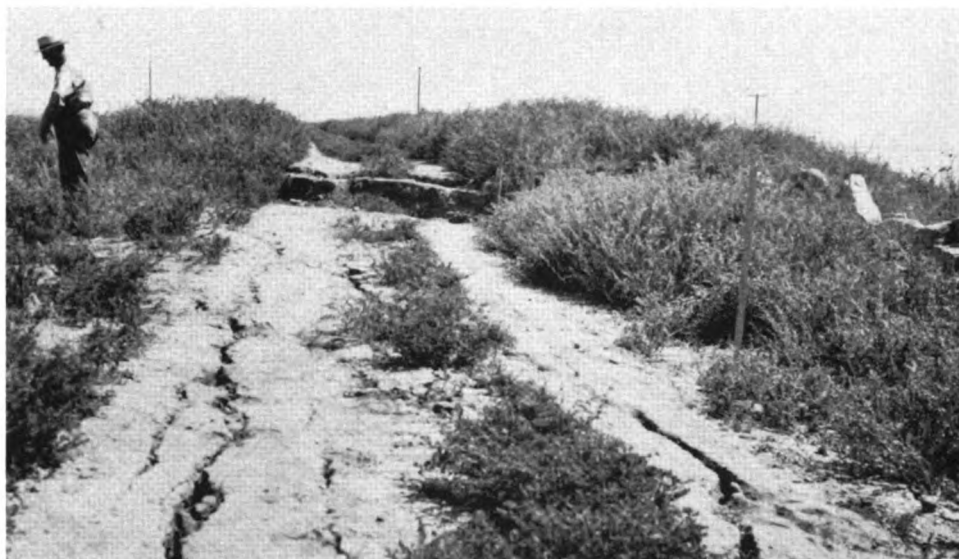
Photo No. 37—Buena Vista Dam No. 732. East levee, looking south. Subsidence and cracking of fill caused by earthquake of July 21, 1952. Maximum settlement of two feet.
