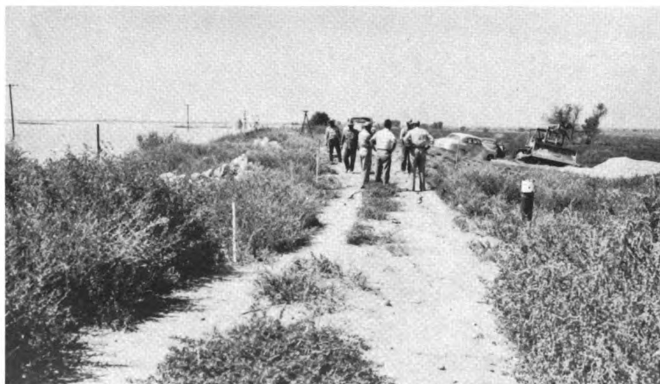
Photo No. 38—Buena Vista Dam No. 732. East levee, looking north. Subsided section of fill. Dozer starting low levee construction using imported stockpiled materials.
