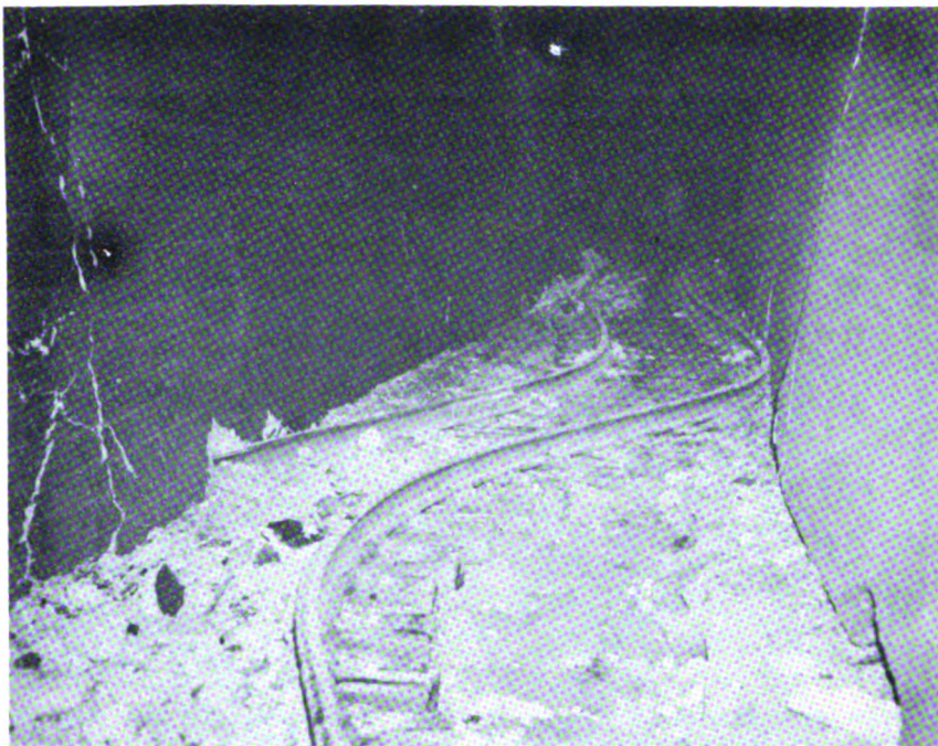
Photo No. 17—Rails and walls buckled by compression in Southern Pacific Tunnel 3 about one mile south of Caliente. Photo by Southern Pacific Company.
