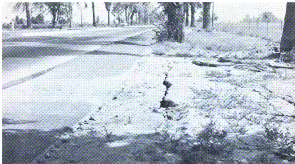
Photo No. 5—U. S. Highway 99 about 10 miles south of Bakersfield. The concrete paved roadway sagged but did not fracture. Photo by Division of Highways.
