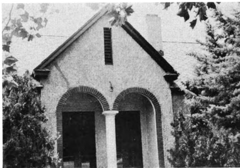
Photo No. 32—Tehachapi school constructed more recently than Cummings Valley school. Though in a center of destruction, the only damage was reopening of a crack above an arch. The original crack was opened by a previous minor earth shock. Photo by Division of Architecture.
