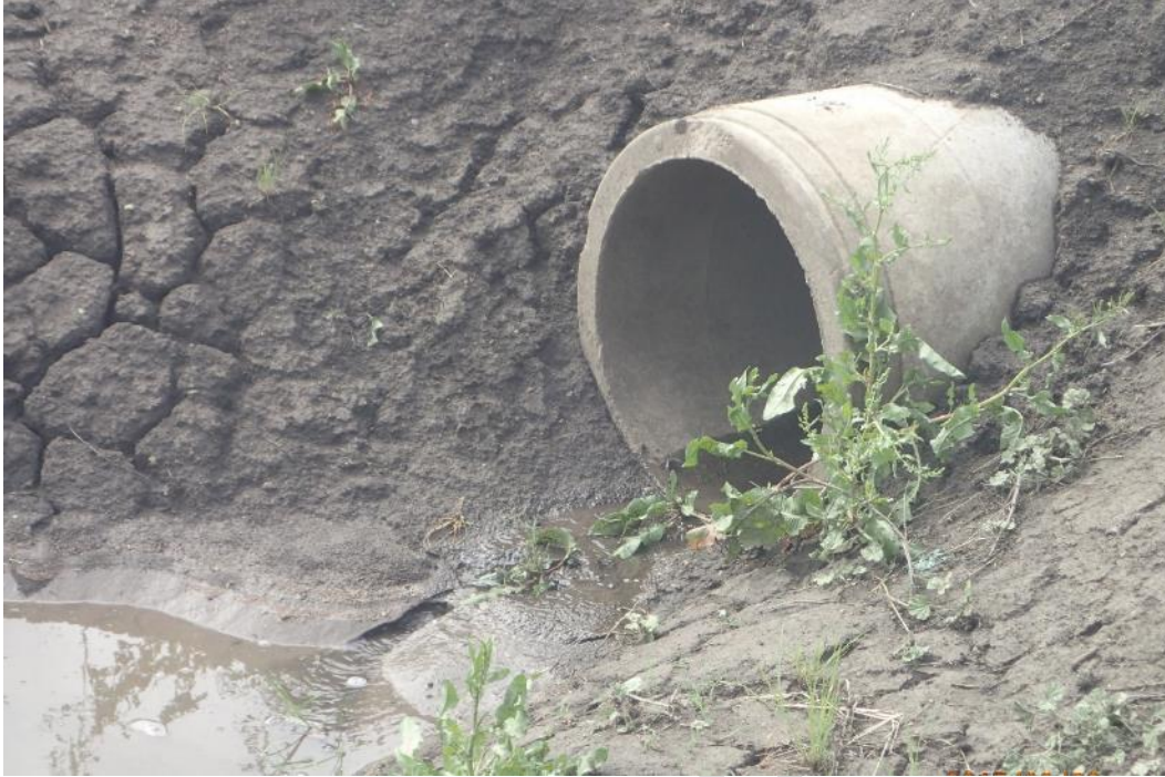
Figure 8 – Small leak from closed canal gate connected to Angelo Canal. Three other gates with similar leaks were observed from Angelo Canal.
