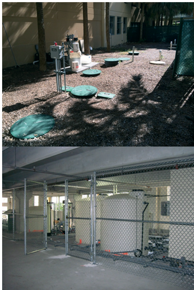
Fig. 2 The UM net-zero water treatment system, 85% recycle rate: (upper panel) below-grade septic tank, membrane bioreactor, and cistern, and (lower panel) UV-hydrogen peroxide advanced oxidation (aerated precipitation/aluminum electrocoagulation/vacuum ultrafiltration not shown).
