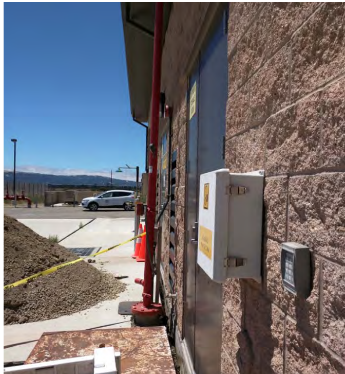
Photo 1: View of an approximate 4-inch separation between south wall of Well House and concrete pad. Note the red fire protection line is also separated from the building at the bottom.
