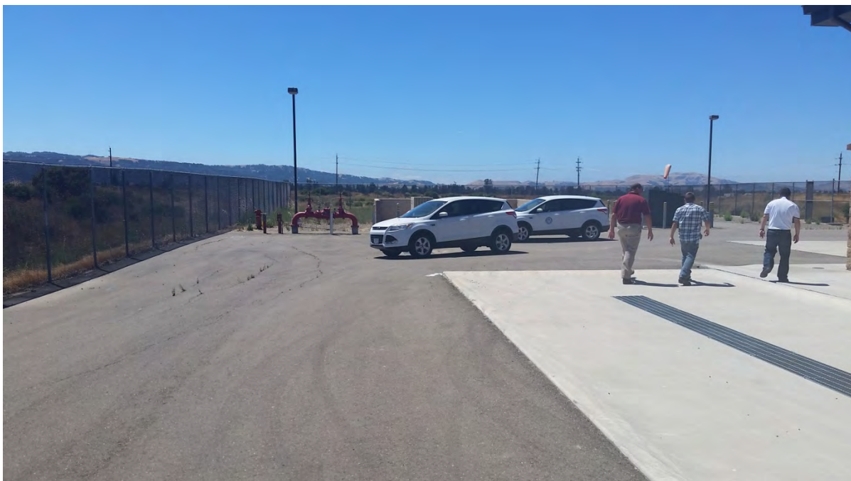
Photo #4: View looking west. Note the arcuate cracks in the asphalt pavement (left of car in the middle of the photo).
