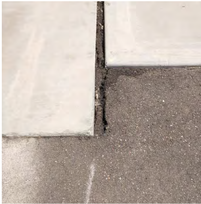
Photo #3: View of separation between the asphalt and concrete pad northwest of the building.
